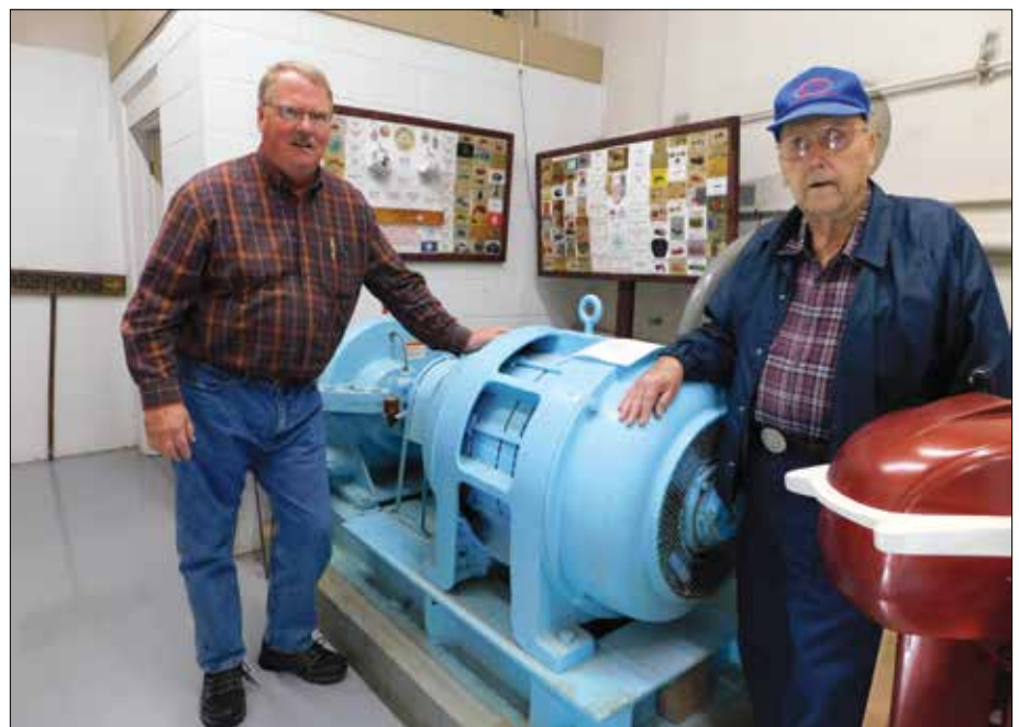
This pump used to provide water to the city from wells beneath the building. (Bob Deck)
